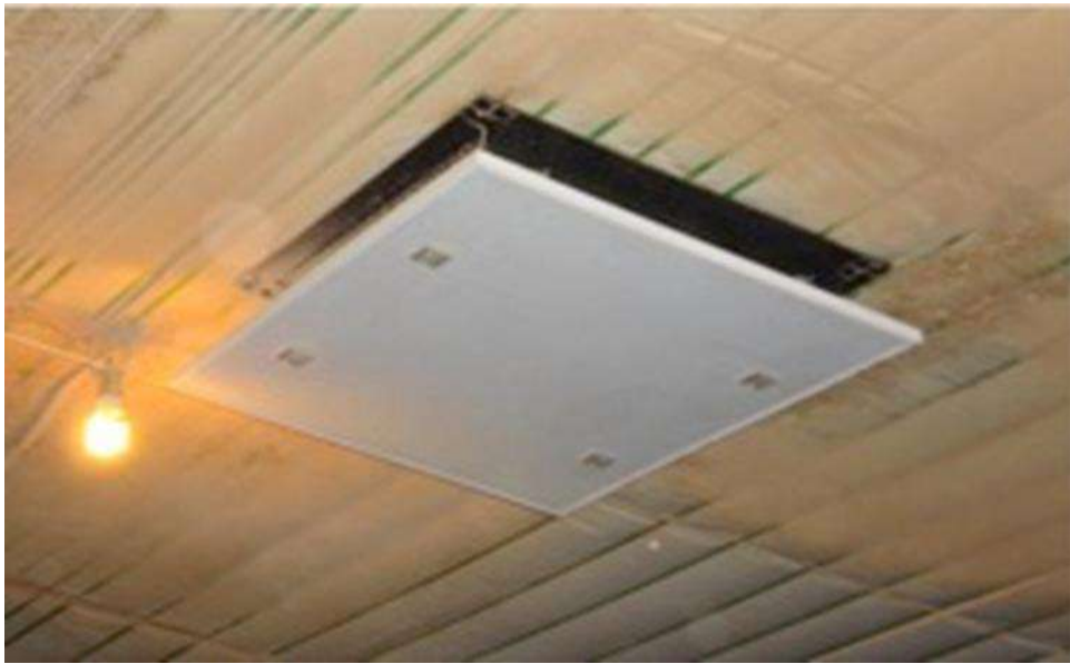
Figure 6. With an insulated attic, the air is warmer than outside air. Using the air allows higher ventilation rates to be used without increasing fuel usage. These increased ventilation rates will help maintain relative humidity between 50 and 70 percent.
